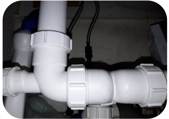
New trap installed
