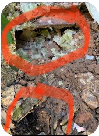
Damage in underground waste pipe system
