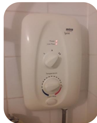
New shower tested working
