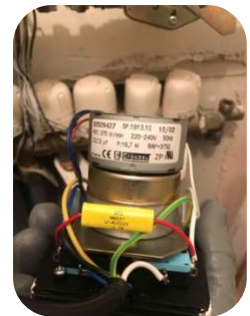
New pump motor installed
