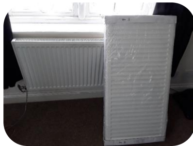
Old & new radiators
