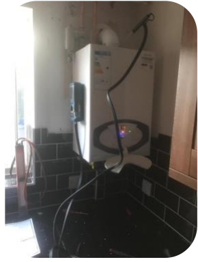
New boiler being commissioned
