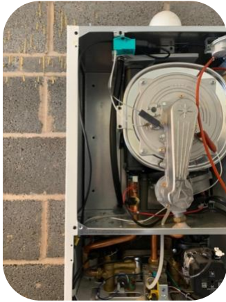
Old expansion vessel removed
