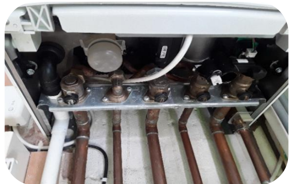
New boiler condensing trap installed
