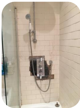
Damage caused by another contractor
