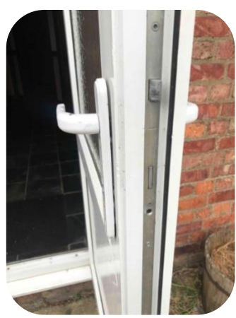
Damaged PVC door lock
