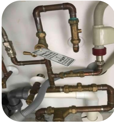
New outside stop valve
