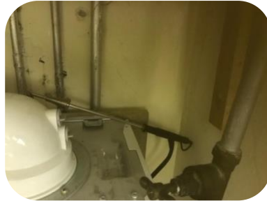
New boiler being tested
