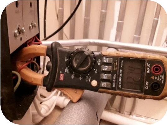
Testing boiler PCB
