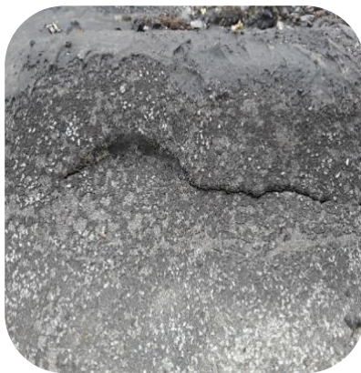
Crack on roof before repair work
