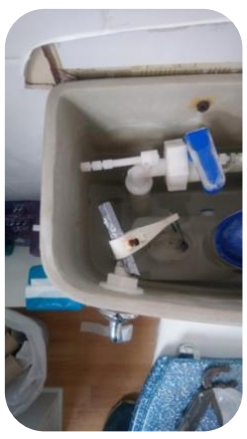
Damaged toilet handle
