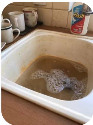
Sink blocked (before work)
