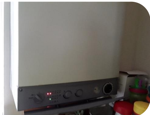
Tested boiler after re-filling system
