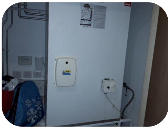
Old boiler before replacement
