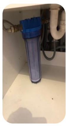
New water filter installed
