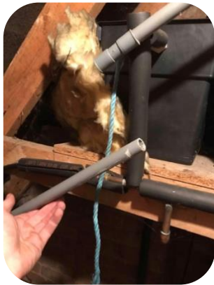
Old snapped overflow pipe
