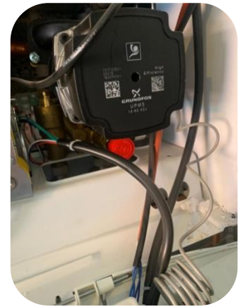
New pump fitted
