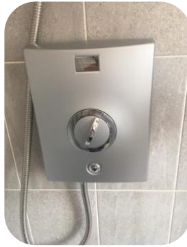
Old faulty electrical shower
