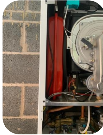
New expansion vessel installed
