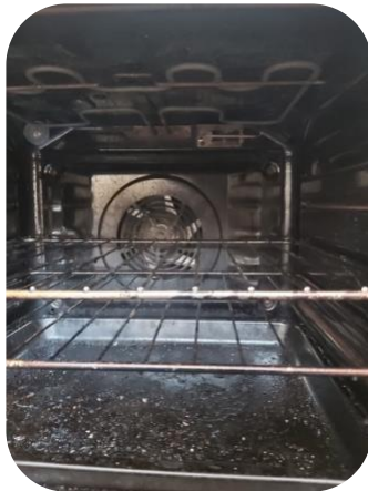
New oven fan & heating element installed
